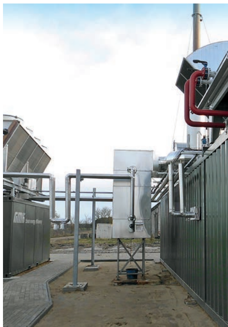
Biogasanlage in Siggelkow.
